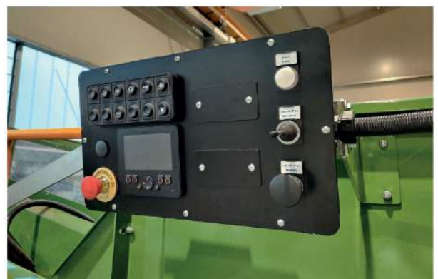
K650 - Control panel
